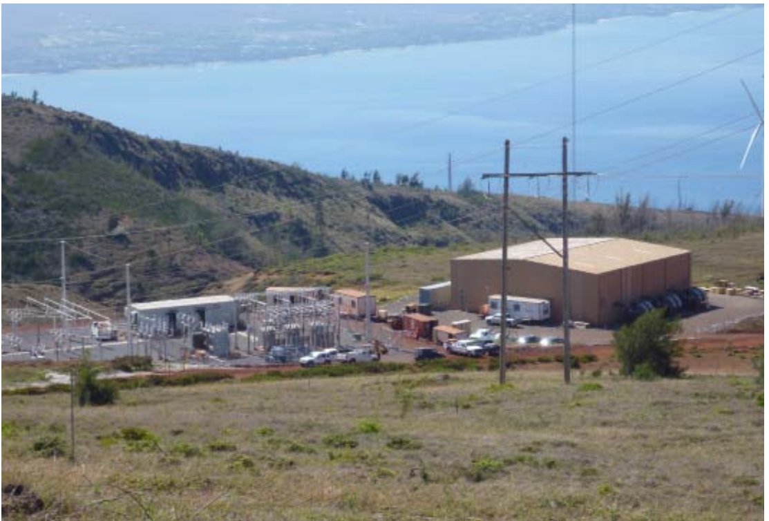
Fig 5: Xtreme Power's integrated power management and energy storage solution is housed at the KWPII site overlooking the Pacific Ocean.
