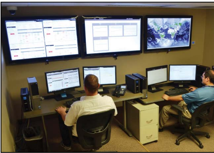
Fig 3: Xtreme Power's 24/7 Operations Center allows Xtreme Power's engineers to monitor all field installations remotely and analyze the DPR®'s performance in Real-time.
