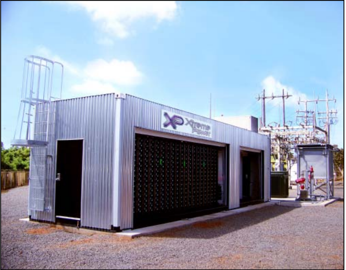
Fig 2: Xtreme Power's containerized Dynamic Power Resource® (DPR®) with 1.5 MVA rated capacity and 15 minutes of energy storage duration.
