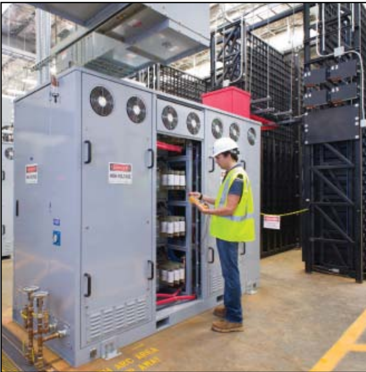
Fig 6: A shot inside Xtreme Power's 15 MVA rated DPR® at Kahuku installation on the island of Oahu, HI, First Wind's second project with Xtreme Power.
