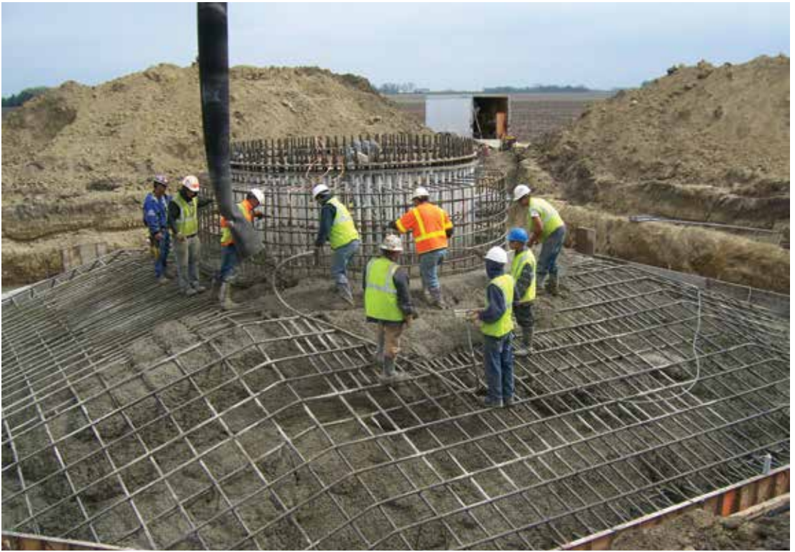
Figure 3: Concrete crew places concrete on the base section of a spread footing foundation.
