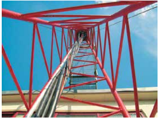
Figure 3: A view at the HELUKABEL wind cable test tower. Up to 20 cables can be tested at once under conditions found in wind turbines located throughout the world.
