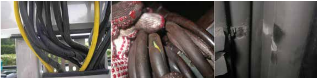
Figure 4: Wind cable performance can be reduced in part by exposure to extreme temperatures, oils and other lubricants, and mechanical stress. It's important to select cables that can withstand these and other challenges within the turbine for long-lasting cable performance.
