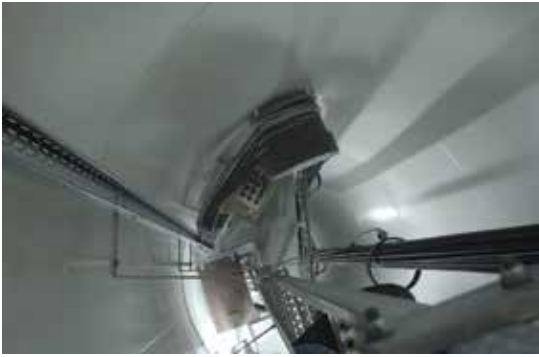
Figure 1: A view of the tower and loop cables of a wind turbine.
