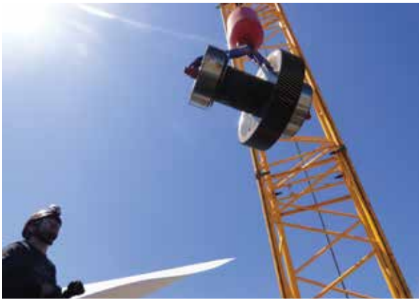
Photo taken during the up-tower gearbox repair to replace the intermediate speed shaft bearings.
