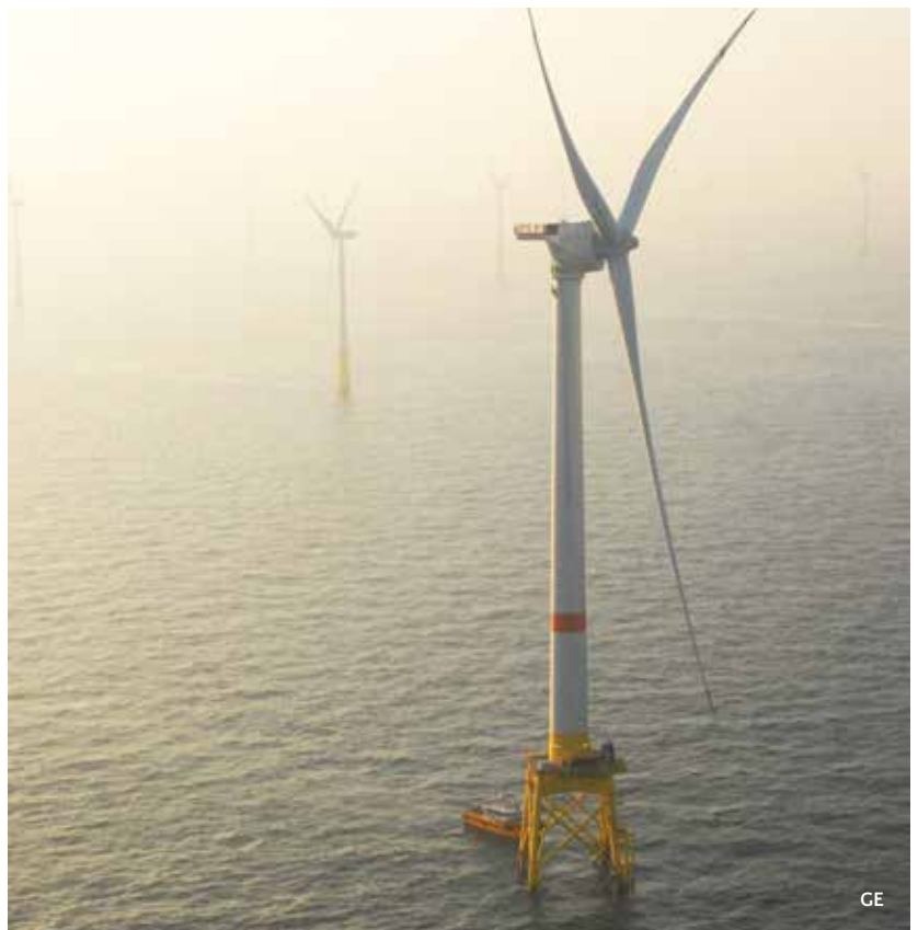
The massive Haliade turbine has a rotor diameter of 150 meters. It can generate 6 MW.
